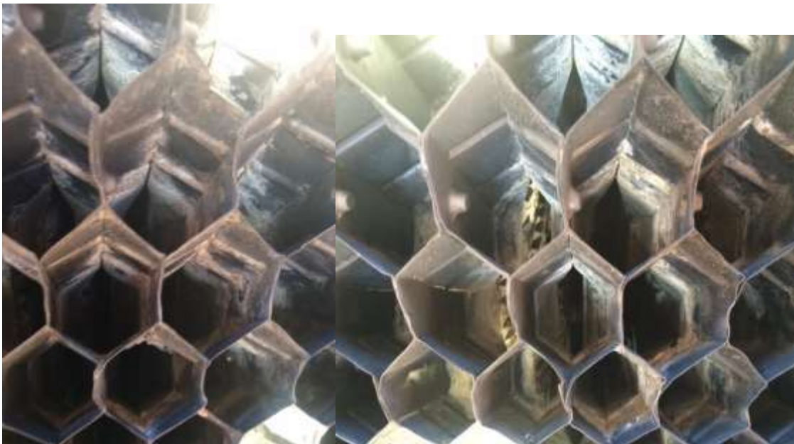
Before pictures of the Cooling Tower fins.
